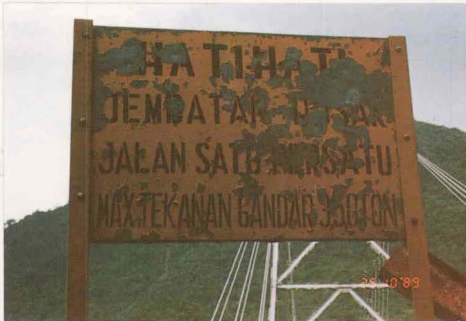
Figure A4.80 - Axle Load Sign in Poor Condition Routine Maintenance Required
