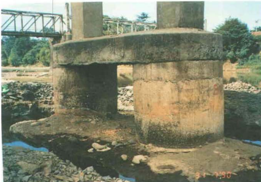
Figure A4.6 - Foundation Type SU Caisson (Note Excessive Stream Degredation)
