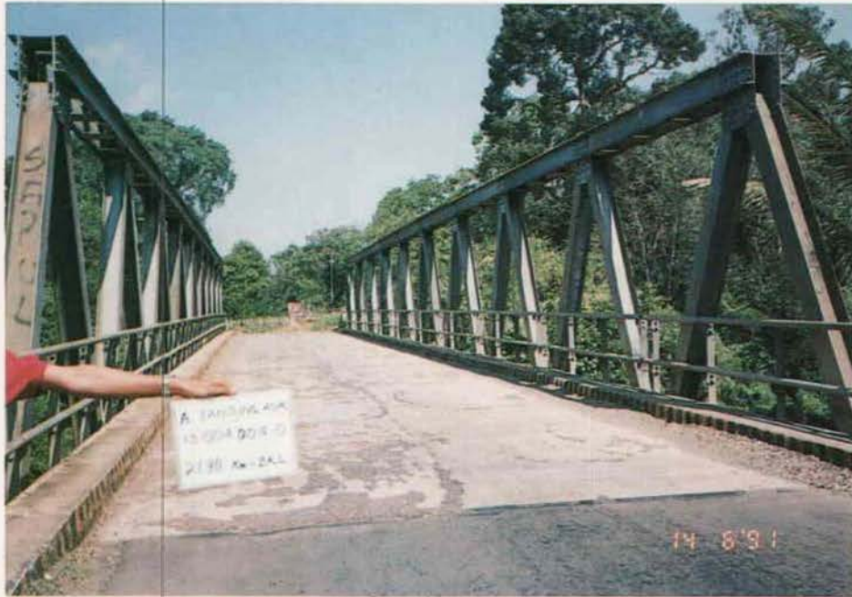
Figure A4.42 - Superstructure Type RBB New Dutch Steel Truss (Short Spans with no Verticals)
