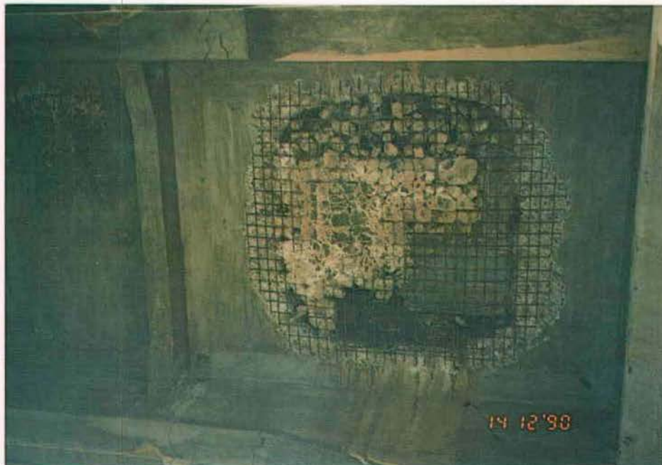
Figure A4.55 - Dangerous Deck Condition Emergency Action Required
