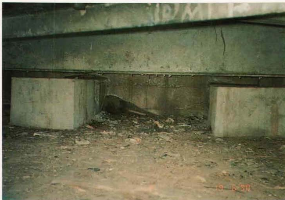
Figure A4.88 - Missing Earthquake Restraint at Abutment 2
