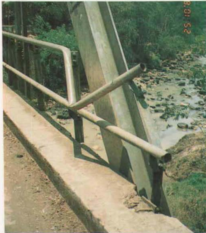
Figure A4.78 - Minor Repairs to Handrails Required
