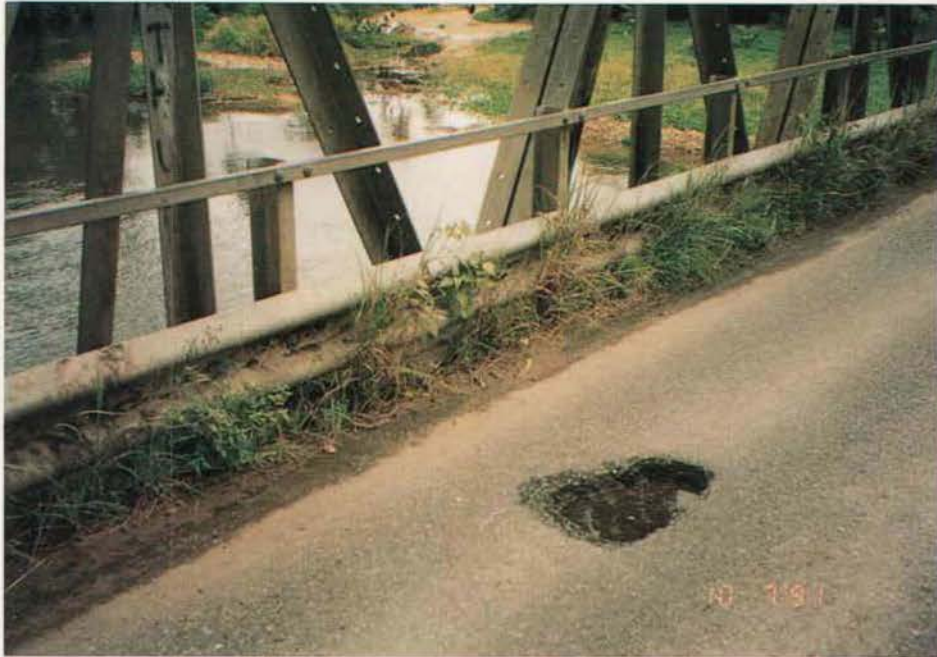
Figure A4.76 - Pot Hole in Deck and Dirt and Vegetation along Kerb needs minor repairs and cleaning
