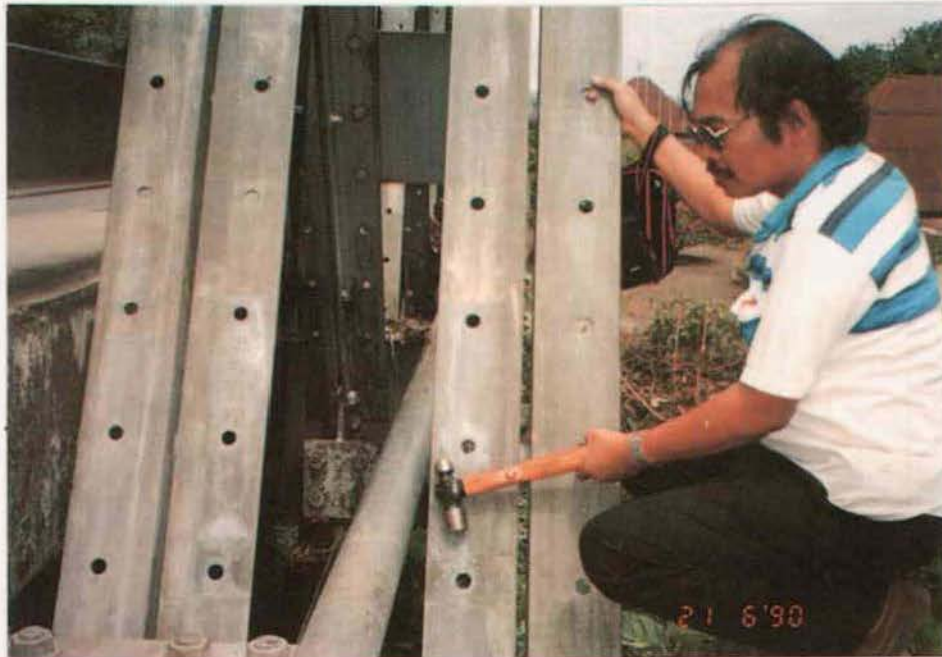
Figure A4.90 - Missing Gusset Plate
