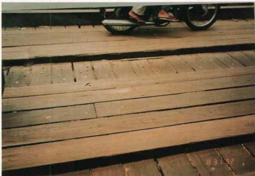
Figure A4.75 - Example of Good Routine Maintenance with Well Maintained Timber Deck Planks
