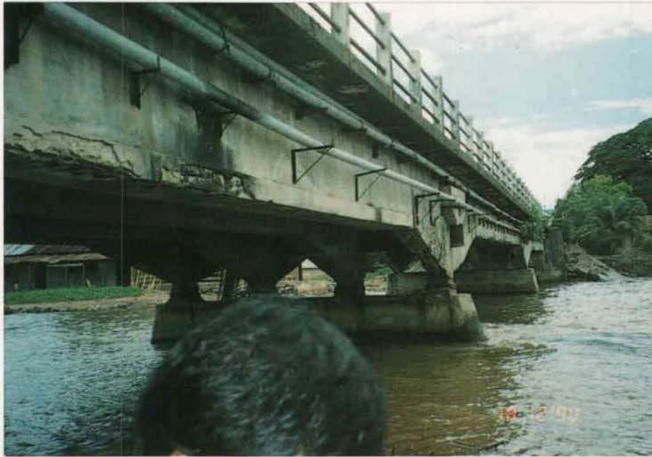
Figure A4.92 - Concrete girder system all in poor condition due to very poor quality concrete
