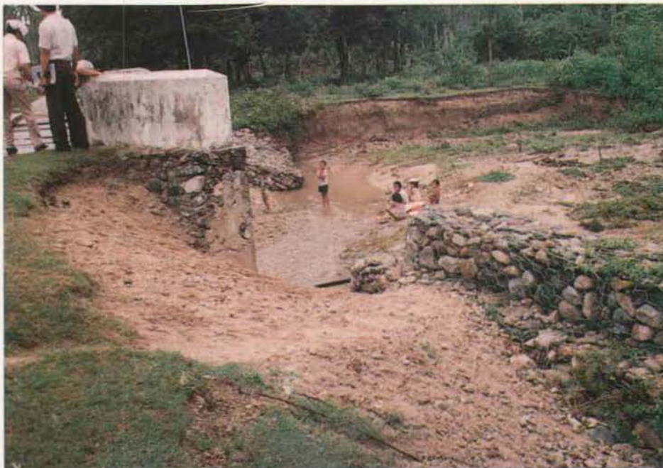
Figure A4.79 - Poor Bridge Approach Drainage Causing Scouring
