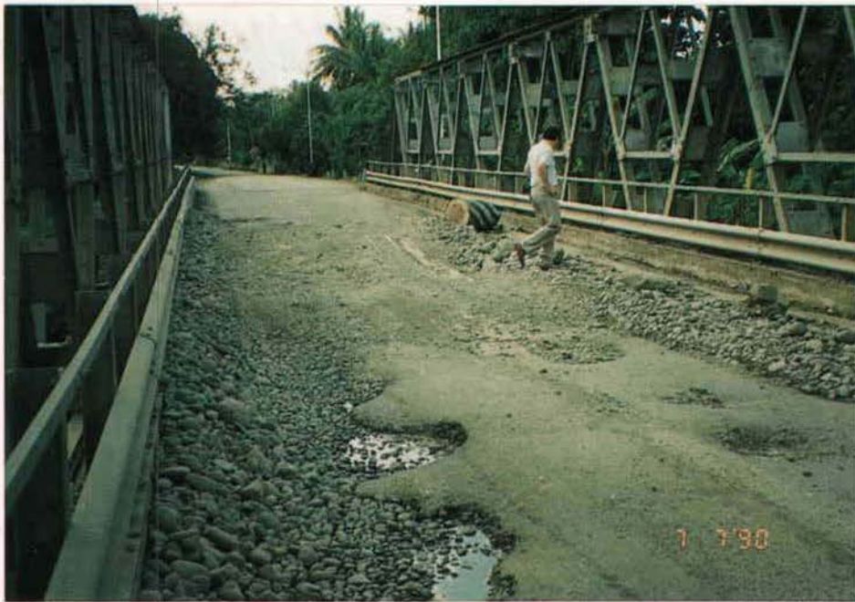
Figure A4.54 - Dangerous Deck Condition Emergency Action Required
