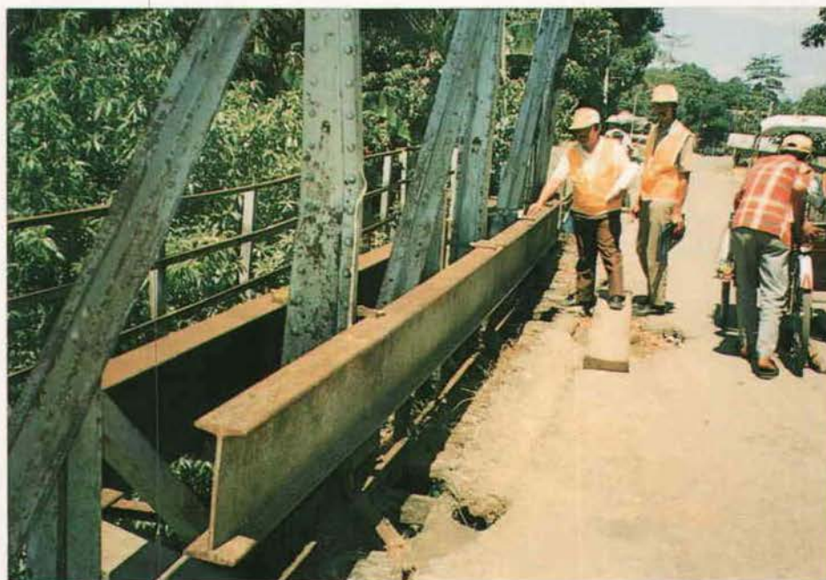
Figure A4.61 - Extra Girder Used to Redistribute Load Across Damaged Truss Section
