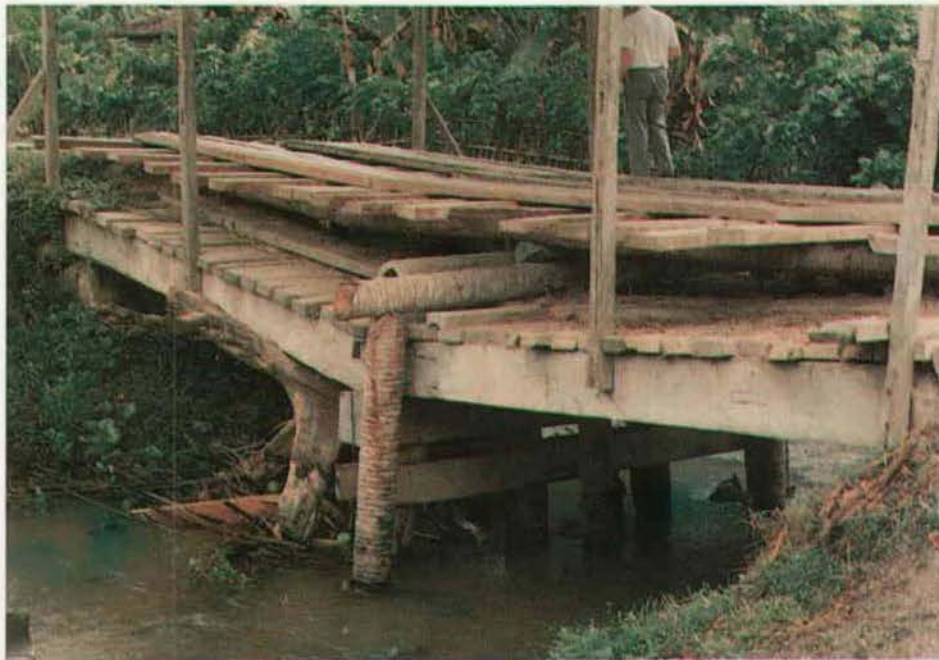
Figure A4.85 - Foundation Settlement at Pier
