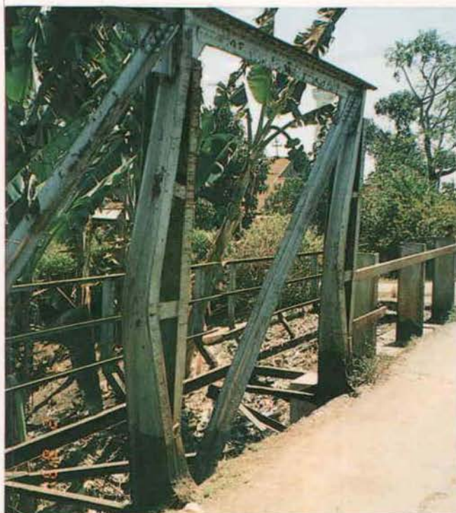
Figure A4.60 - Damaged Truss Vertical Strengthened
