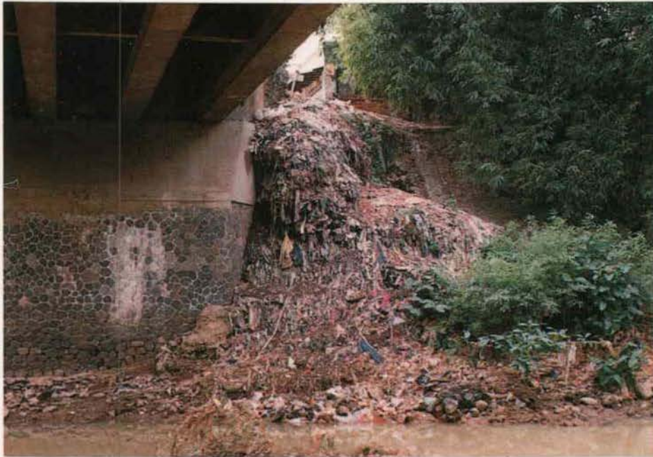
Figure A4.66 - Rubbish and Debris Need Removal Routine Maintenance Required
