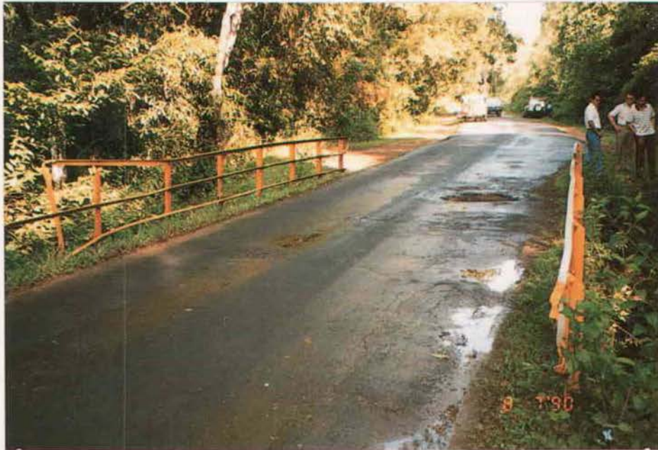
Figure A4.74 - Potholed Deck needs minor repairs
