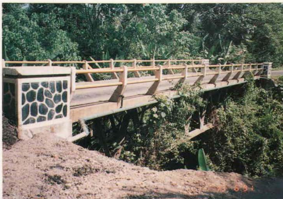
Figure A4.71 - Excessive Vegetation in Trusses Routine Maintenance Required
