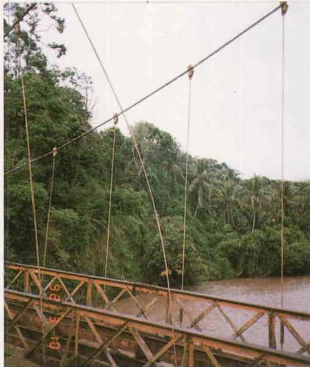
Figure A4.64 - Unsecured Hangers on Suspension Bridge Emergency Action Required
