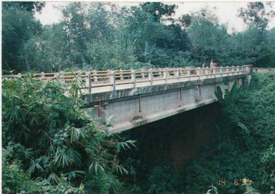
Figure A4.96 - Scuppers too short directing water onto girder
