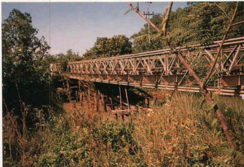
Figure A4.38 - Superstructure Type RBW/SBW Bailey Type Steel Truss Bridge (Acrow Type)
