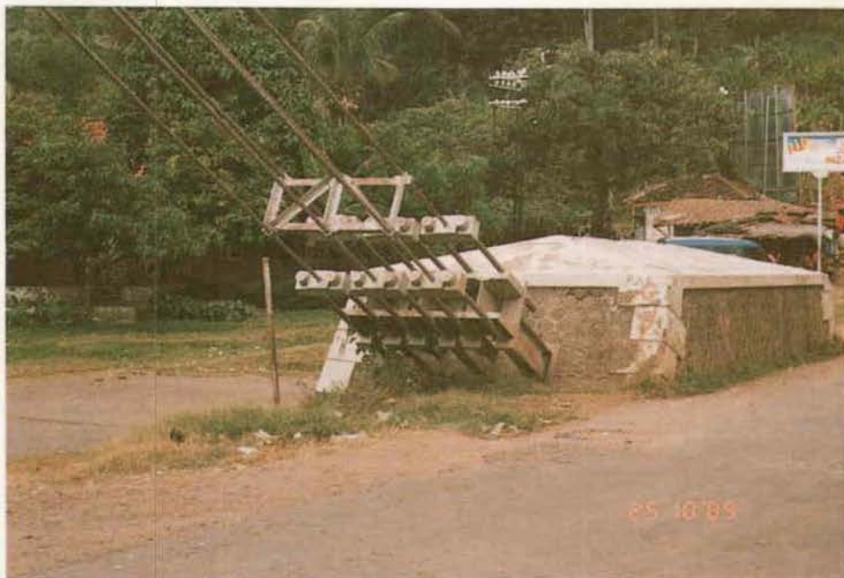
Figure A4.69 - Example of Good Routine Maintenance Keeping the Anchor Area at a Suspension Bridge Clean
