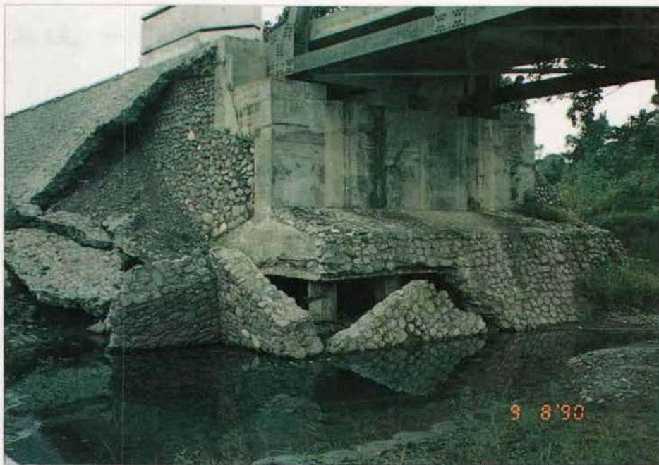
Figure A4.84 - Scour at Abutment 1
