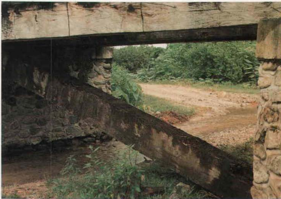
Figure A4.95 - Collapsed Girder
