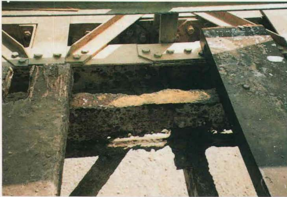
Figure A4.99 - All Steel Deck Stringers Corroded in Span 1
