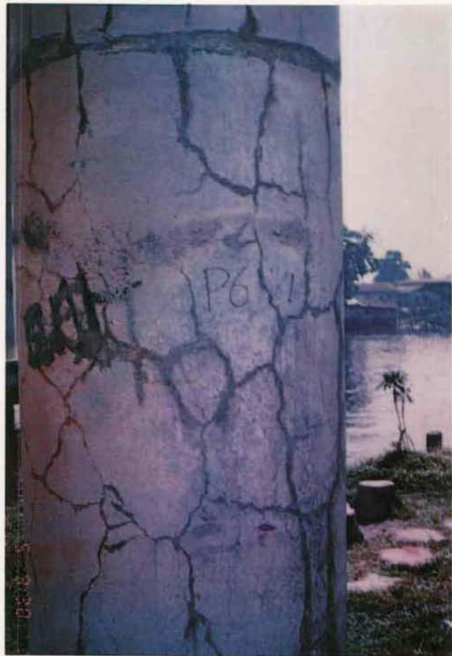
Figure A4.87 - All Columns in Pier 6 Extensively Cracked
