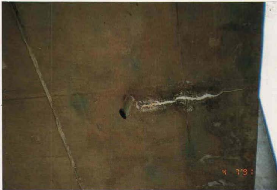
Figure A4.101 - Isolated Crack in Concrete Deck Span 2
