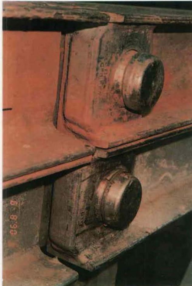
Figure A4.89 - Bridge Circlip Missing at 5th Panel on Chord on Left Side of Bridge
