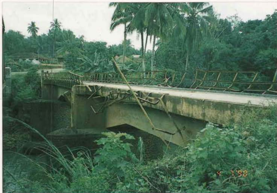
Figure A4.51 - Missing Handrails on Narrow Bridge Emergency Action Required
