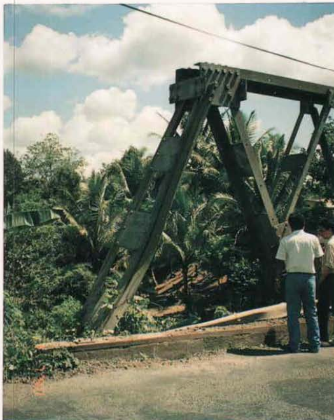
Figure A4.63 - Diagonal of RBU Truss Damaged by Impact
