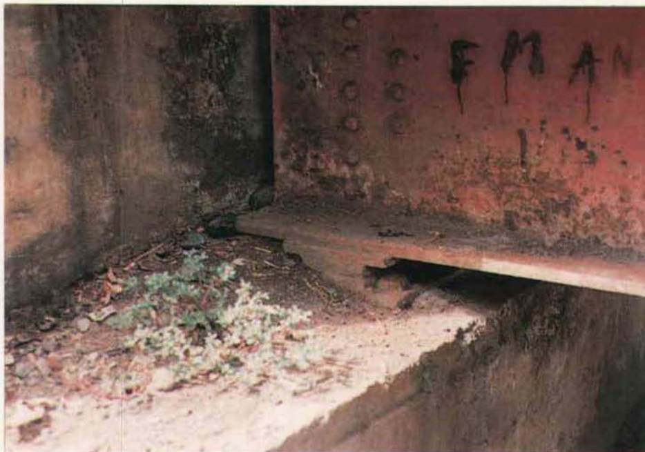
Figure A4.70 - Dirty Crossheads and Bearings Routine Maintenance Required
