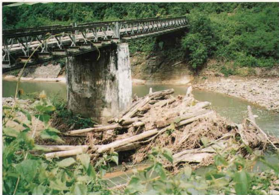
Figure A4.73 - Debris needs to be cleared
