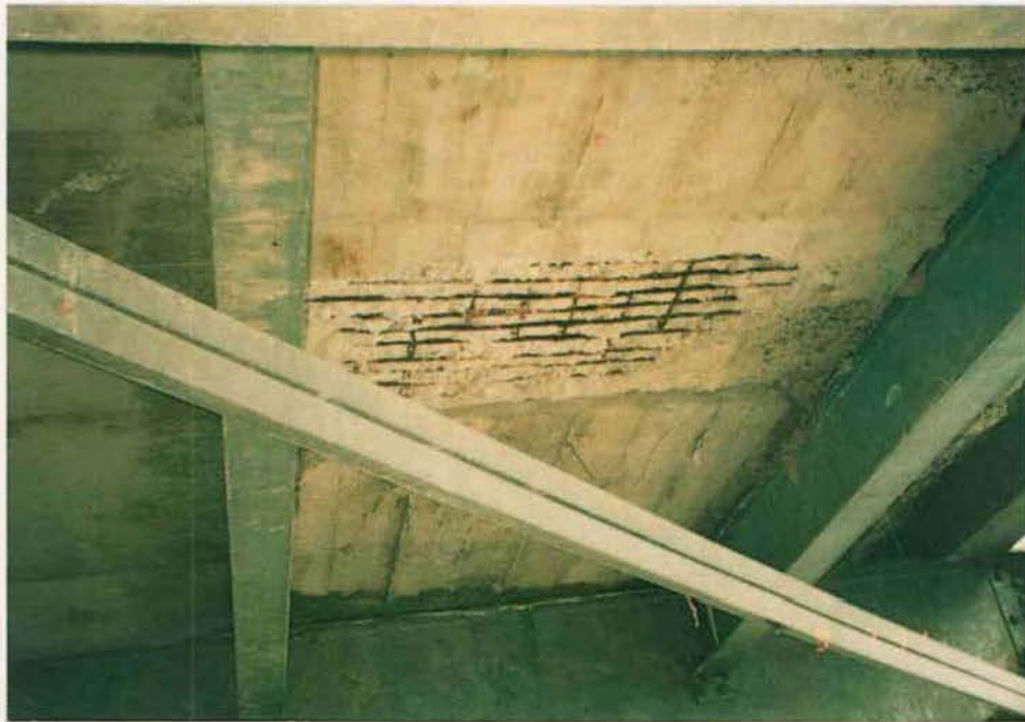
Figure A4.100 - Concrete Spalling under Deck Slab Small Area
