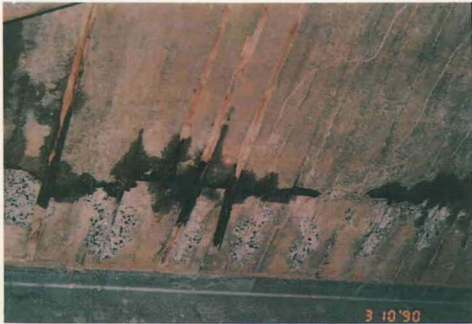
Figure A4.98 - Extensively Cracked Deck
