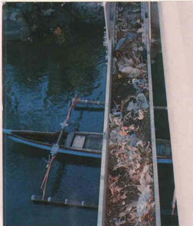
Figure A4.67 - Rubbish in Bottom Chord of Truss can accelerate corrosion Routine Maintenance Required
