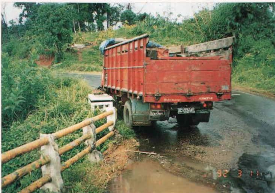
Figure A4.77 - Poor Deck Drainage Routine Maintenance Required
