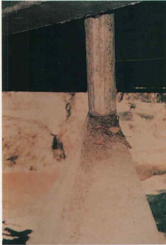
Figure A4.97 - Blocked Scuppers Causing Flooding on Deck
