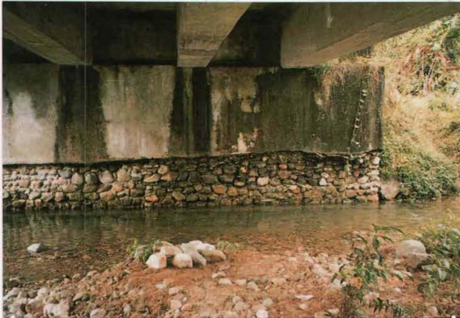
Figure A4.82 - General Degrading of Stream Bed
