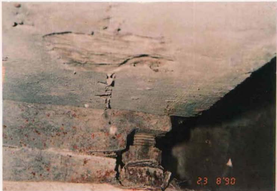
Figure A4.102 - All Bearings Jammed because bolts are too long
