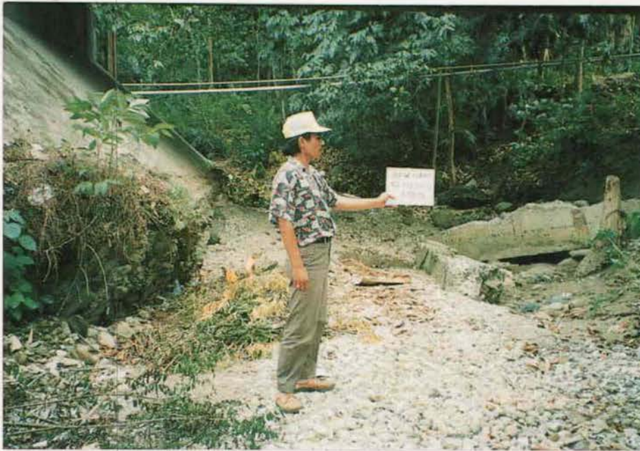
Figure A4.52 - Obstruction, Scour and Stream Degradation
