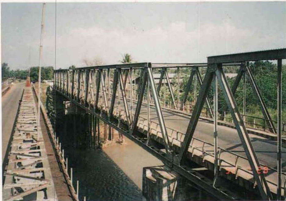
Figure A4.41 - Superstructure Type RBB New Dutch Steel Truss (Long Spans with Verticals)
