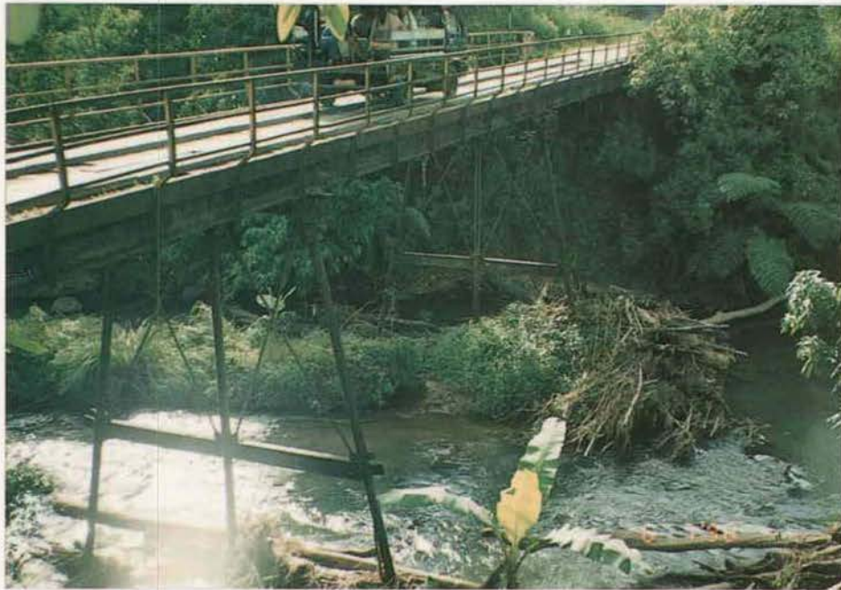
Figure A4.72 - Debris needs to be cleared
