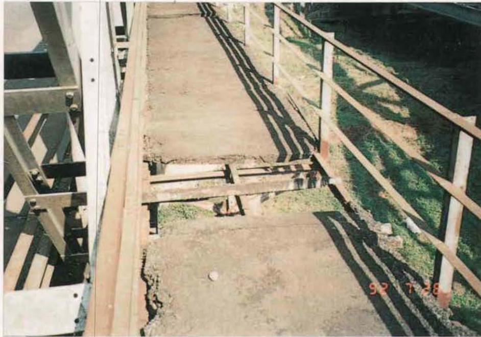
Figure A4.50 - Dangerous Walkway Emergency Action Required
