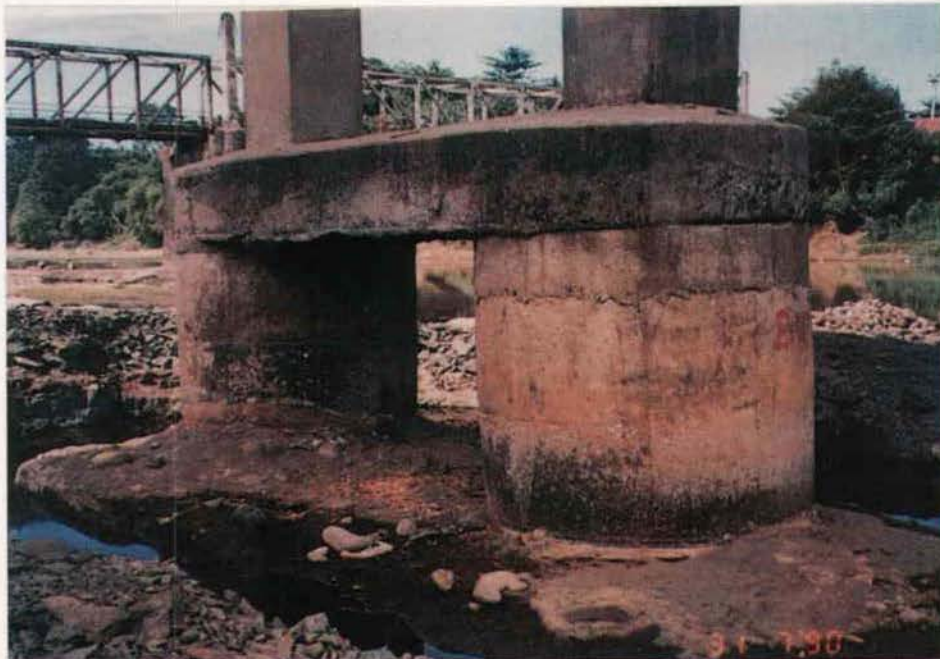
Figure A4.86 - River Bed Degraded Exposing the Caissons and Affecting Stability
