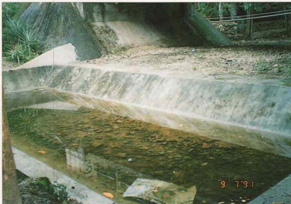
Figure A4.53 - Solution - Bottom Controller Constructed and Stream Bed Returns to Original Bed Level
