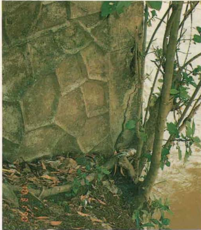
Figure A4.68 - Excessive Vegetation causing cracking of masonry Routine Maintenance Required
