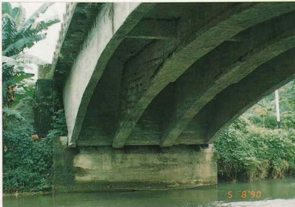
Figure A4.93 - All Concrete Girders with Extensive Spalling
